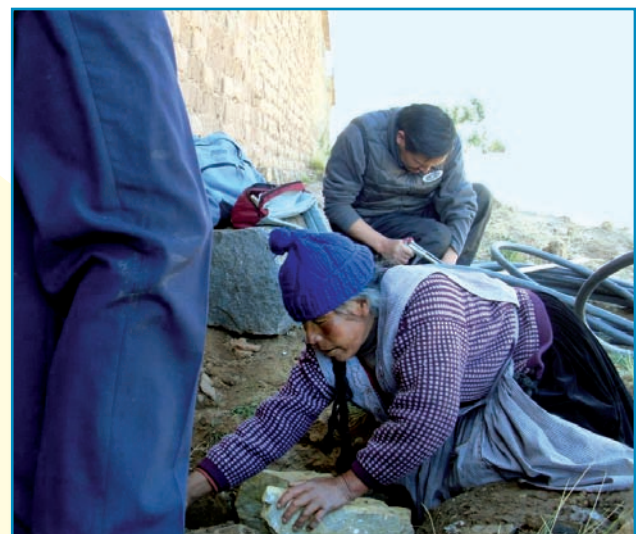
The children (or their parents) who profit from our projects work themselves on these projects, as shown here during the laying of the water pipeline in Chiutara Baja.
